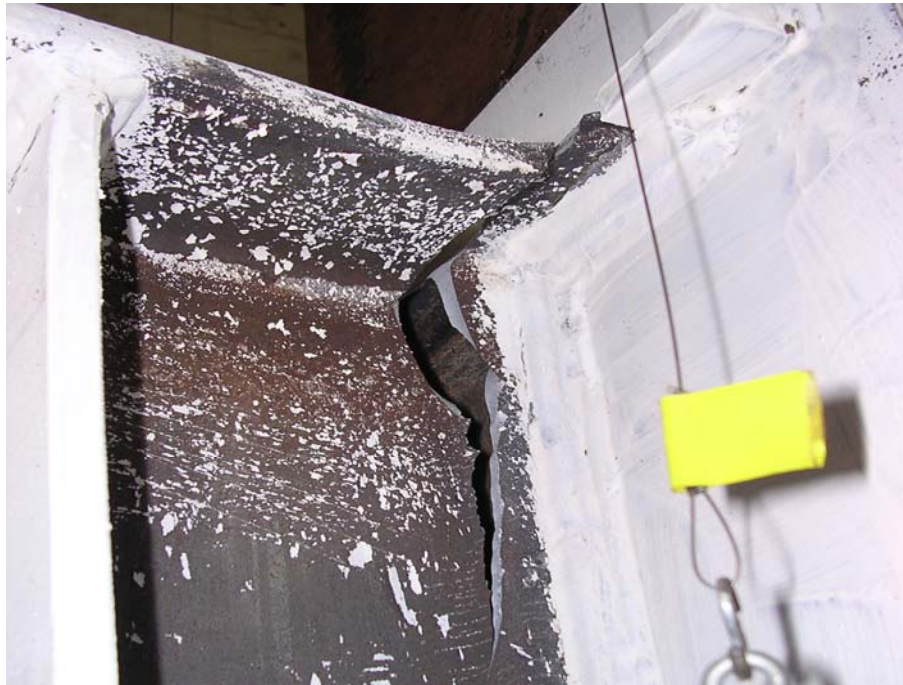
Figure 3.5: Extension of link flange fracture to the link web – AISC-1
