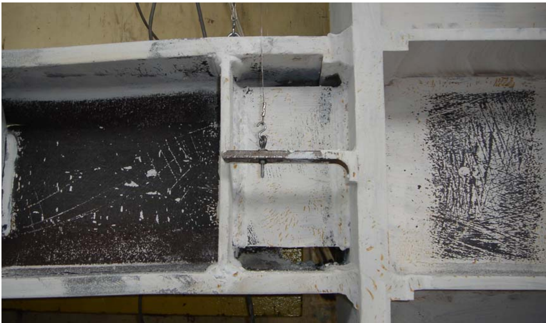
Figure 3.48: No apparent distress in the Link-to-Column Connection after Failure of Specimen AISC-7 during Loading Cycle of \gamma = + 0.12 / - 0.13 rad
