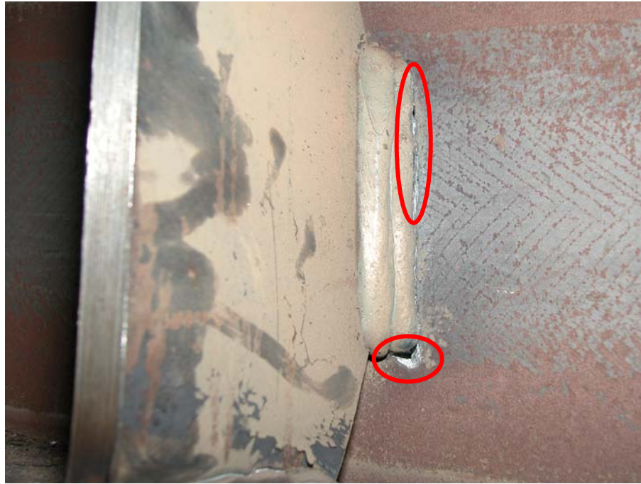
Figure 3.17: Specimen AISC-4 – Web Cracks adjacent to stiffener welds after loading cycle at \gamma = \pm 0.11 rad
