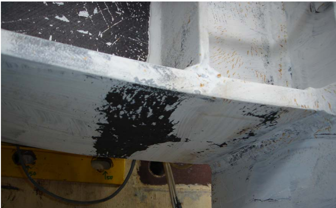
Figure 3.44: Link Bottom Flange at the Link-to-Column Connection after cycle of \gamma = \pm 0.11 rad (Last full loading cycle prior to failure)
