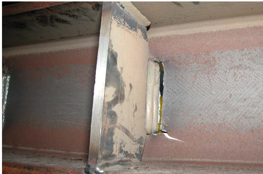
Figure 3.18: Fracture of Link Web adjacent to stiffener's weld during loading cycle of \gamma = + 0.13 rad
